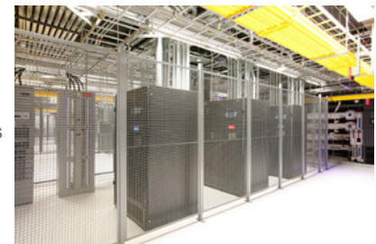
Equinix PH1 IBX data center interior
